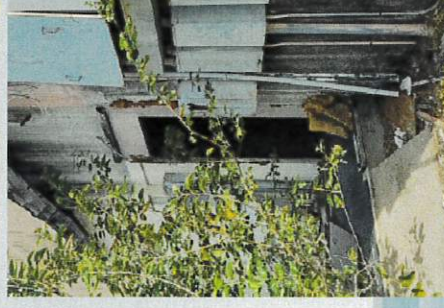
Sections of roof are completely missing.
