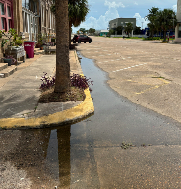
Figure 4.2 | Localized flooding on downtown streets
