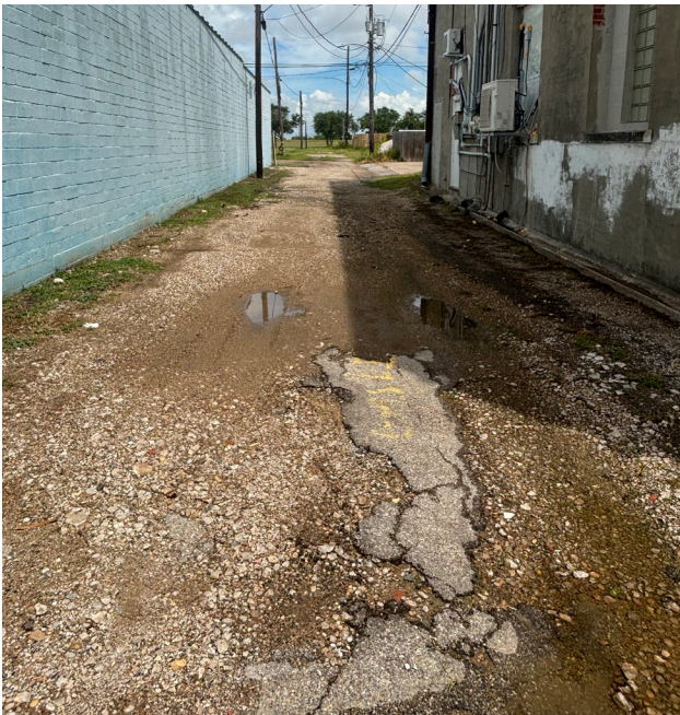
Figure 4.1 | Unpaved alleys create a maintenance issue downtown
