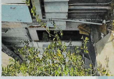
Sections of roof are completely missing.
